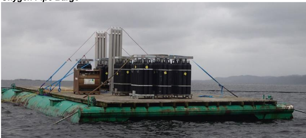
Oxygen Pipe Barge
